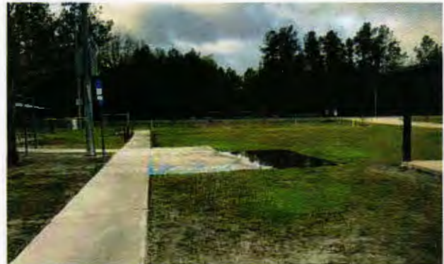
Drainage issues at Kristen M. Higginbotham Sports Complex (top) and Melissa Lynn Raulerson Sports Complex (bottom)
