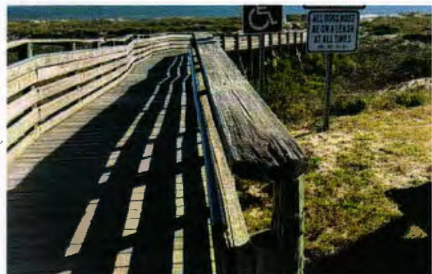
Weathered boardwalk at Burney Park
