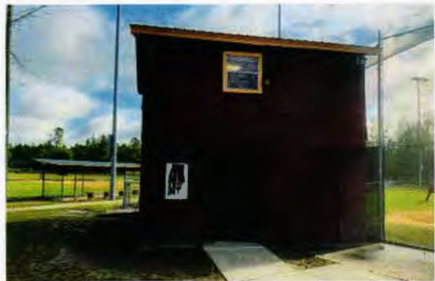
Buildings in need of repair at Stein-Tompkins Sports Complex
